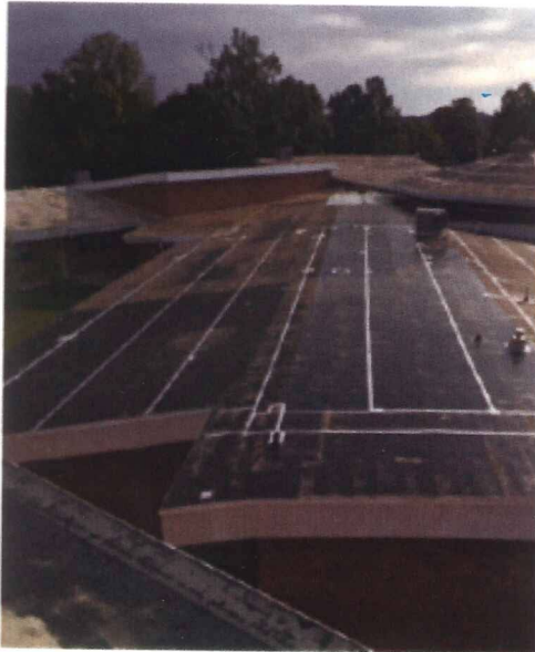
This overview shows the seam tape application, the new flashing in edge, and the moisture still on the roof. This photo was taken at ar
