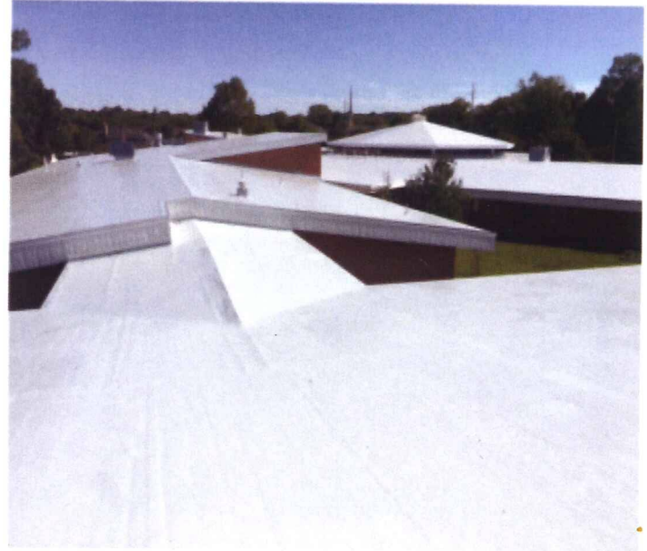
This is just an overview photograph showing the new look. As expected, you can see the seams, flashing, and all undulations through the coating up close, but from the ground it is very smooth.
