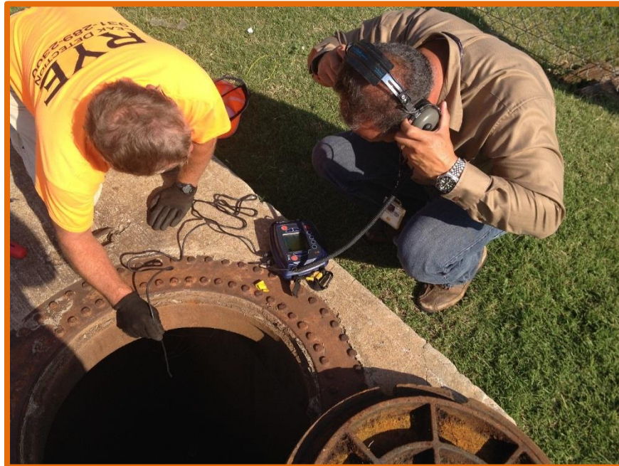
Figure 1. Comprehensive leak detection surveys are a specialty of Rye Engineering PLC. Our crews are fully equipped with the latest technology for leak detection including this handheld listening probe used for localizing leakage.
