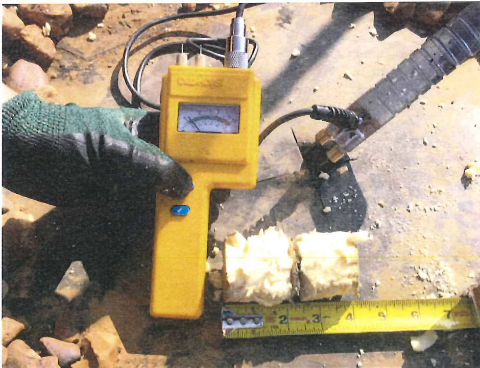
A core sample was taken on this roof system to determine whether the roof system was wet or dry. The moisture gauge was then used to determine the amount of moisture being held within the roof assembly. The core sample was dry where tested.
