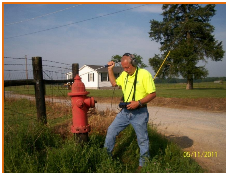
Figure 2. We utilize premium handheld acoustic units to localize leaks by listening to water services, hydrants, etc. and ground microphone attachments to pinpoint leaks for repair.
