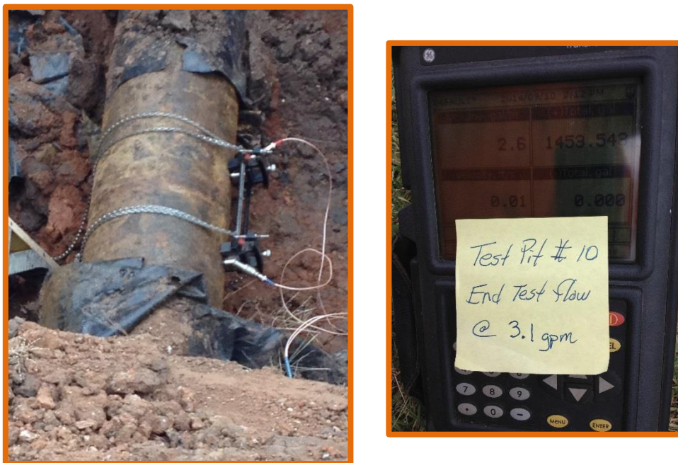
Figure 9. Other Methods – Our crews are experienced in flow-based leak detection methods such as this ultrasonic flow meter which can be attached to the outside of water mains.
