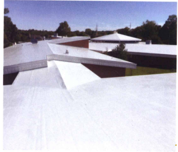
This is just an overview photograph showing the new look. As expected, you can see the seams, flashing, and all undulations through the coating up close, but from the ground it is very smooth.
