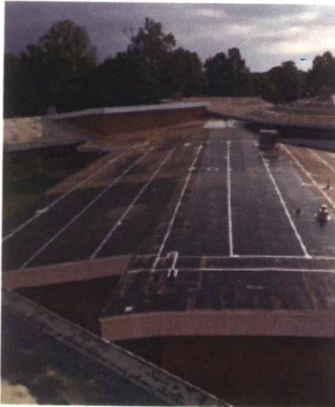
This overview shows the seam tape application, the new flashing in edge, and the moisture still on the roof. This photo was taken at ar
